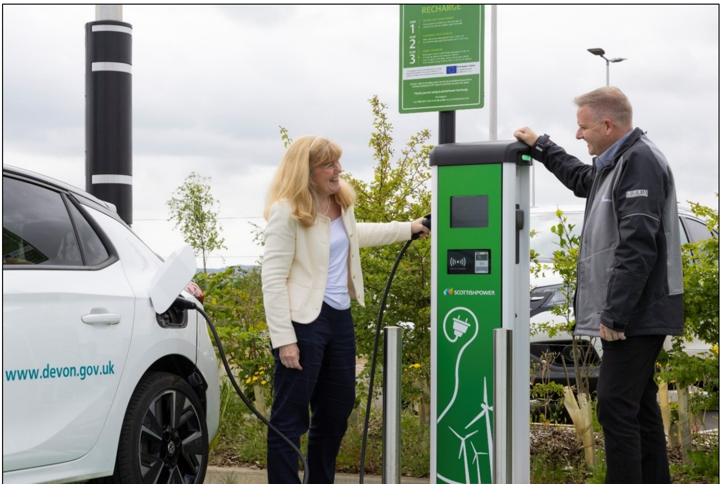
Figure 20 Devon's EV charging infrastructure
